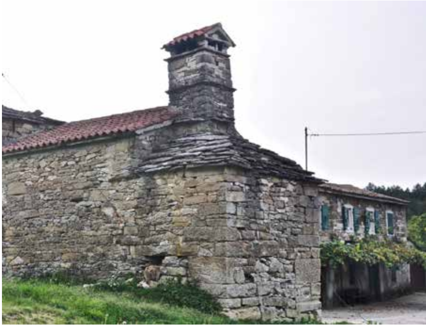
An Istrian spahnjenca – a large alcove opening off the main floorplan of the kitchen, accommodating an open hearth with flue to convey the smoke outside the central room of the house.
